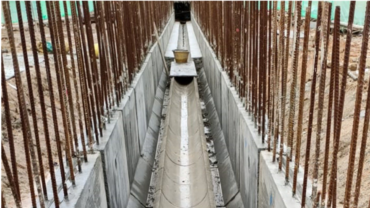
Prototypes of the drain channels have been installed at a JTC construction project near Tuas Link MRT station.
