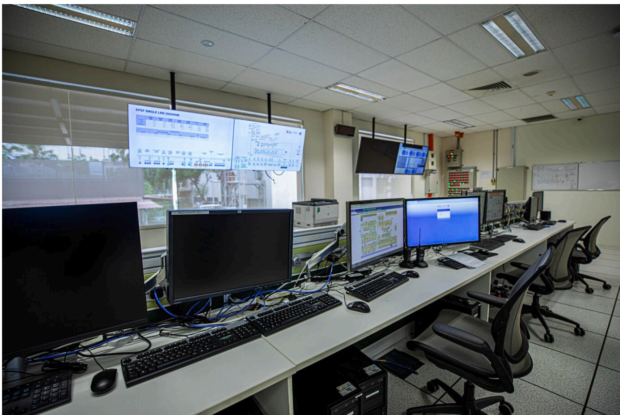
The nucleus of the centre is the control room, which is equipped with automation and intelligence technologies. Here, personnel can perform advanced control and management of grid operations.
