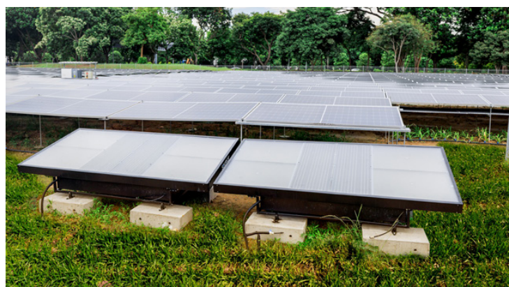
If successful, the hydropanel at Changi Business Park (CBP) could pave the way for more innovative uses to take root at our solar sites.
