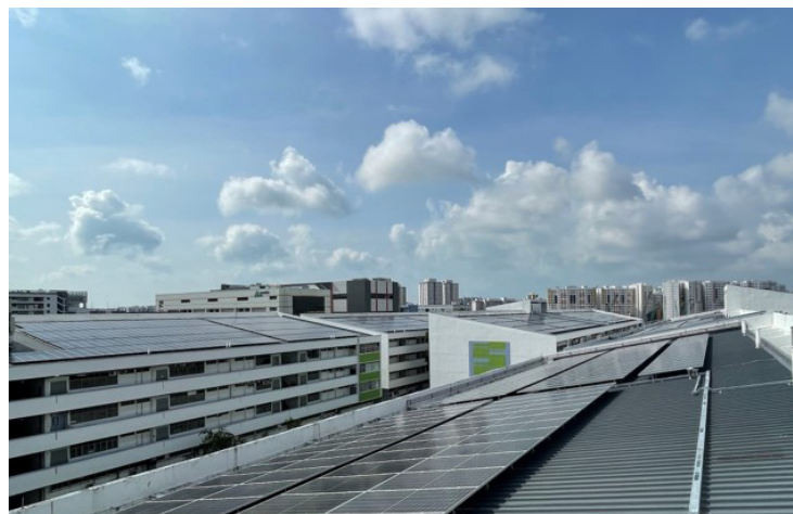
JTC's SolarRoof Programme: Maximising vacant building rooftops for the purpose of generating solar power.
