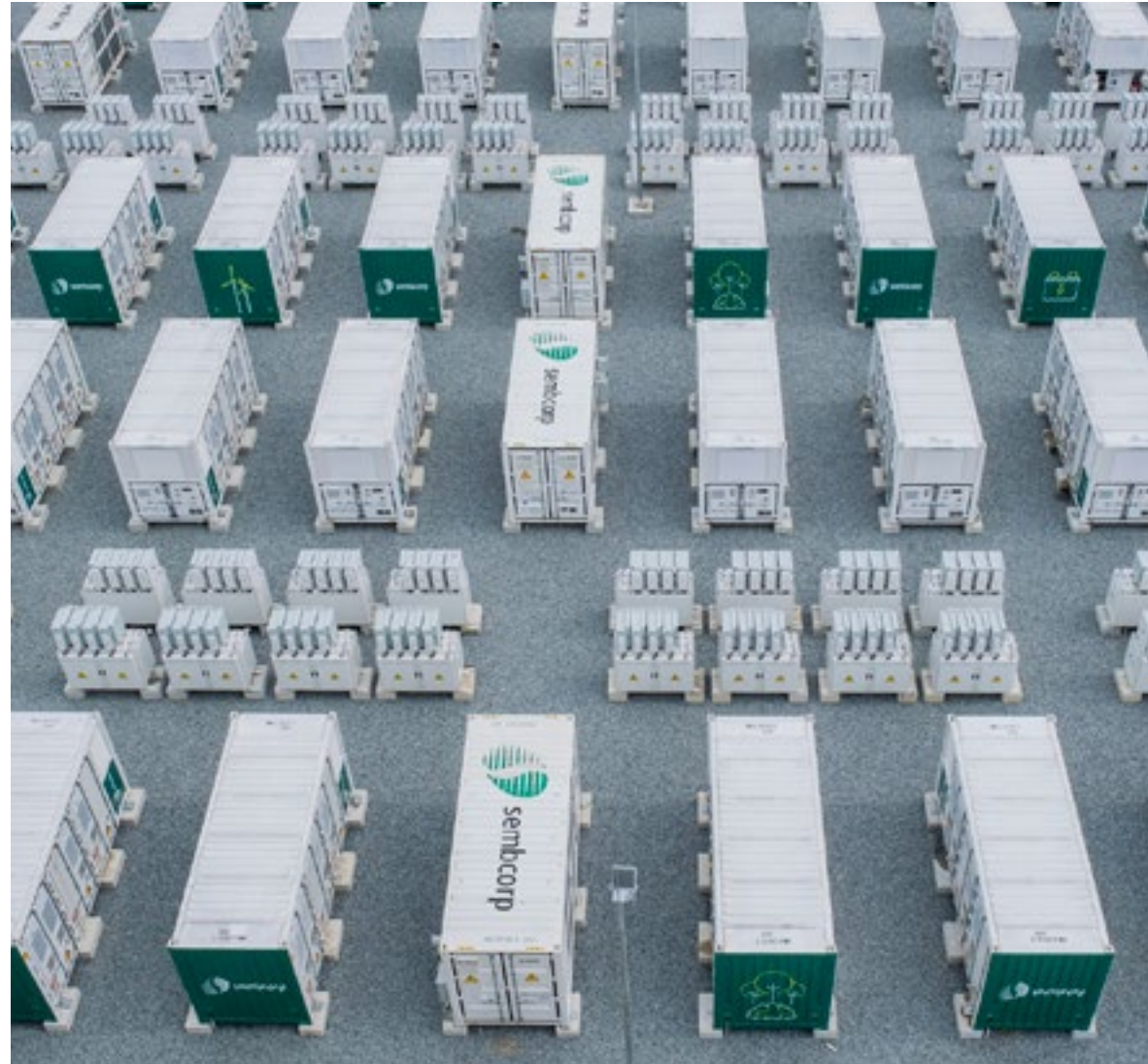
Operational since December 2022, Sembcorp's 285 megawatt-hour (MWh) energy storage system is installed across two sites on Jurong Island: Banyan and Sakra. Photo courtesy of Sembcorp Industries.
